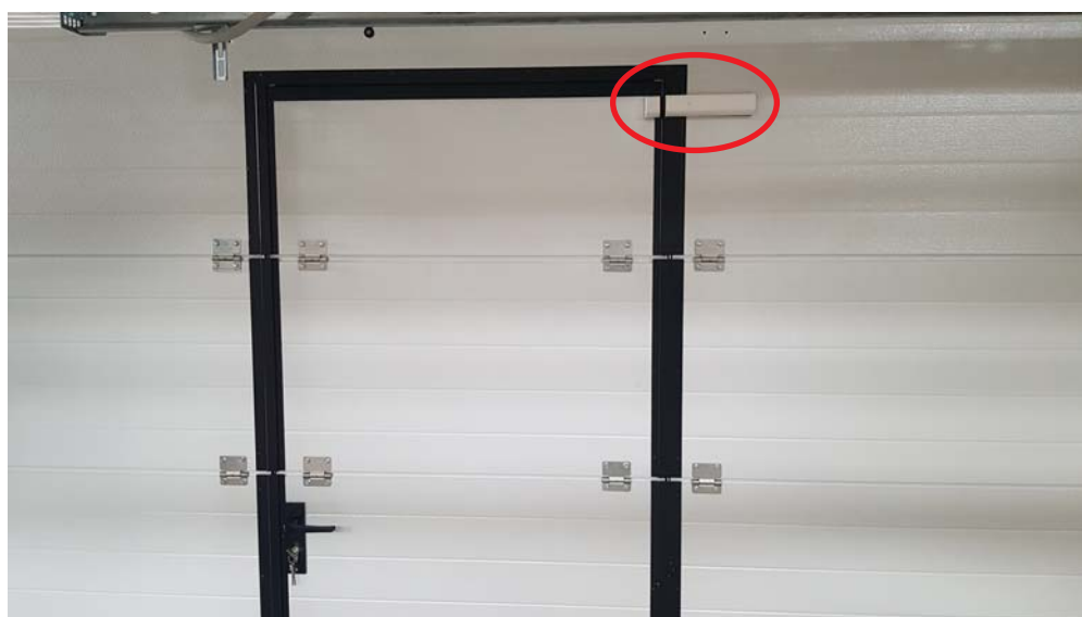
SD01/2 – po instalaci
