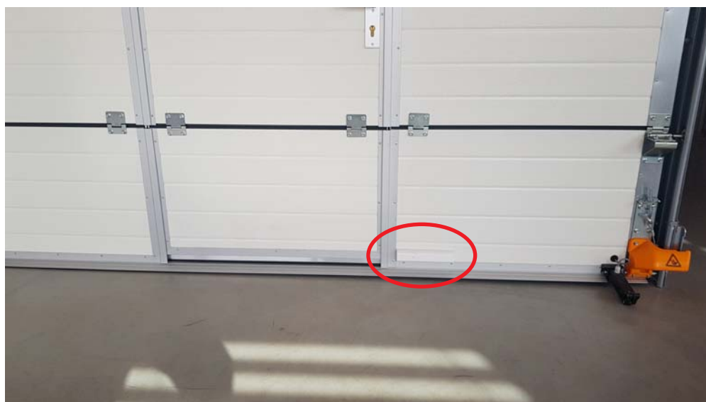
SD01/1 – po instalaci
